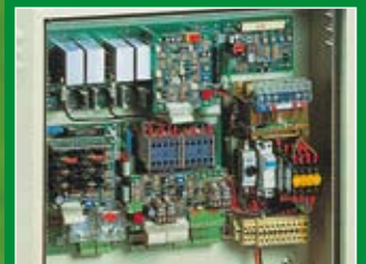
UPS RESCUE DEVICE
